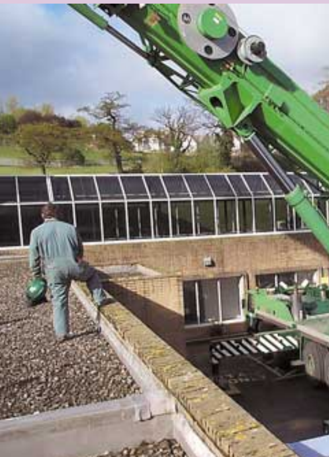
Work in progress on the new custom built unit which now houses the MRI scanner at Perth Royal Infirmary.
